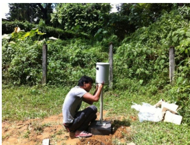
Figure 6.1: Installation of Automatic Rain gauge in Sylhet
