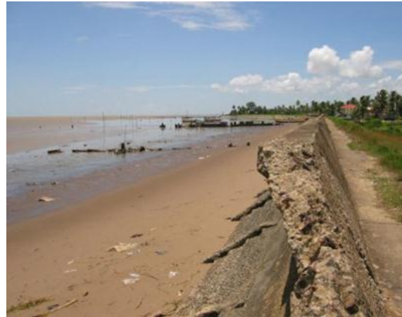
Figure 2. a collapsed structure in British Guyana (photo by H. Winterwerp)
