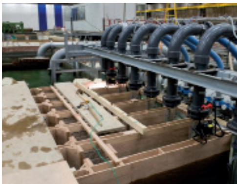
Header for flow withdrawal
