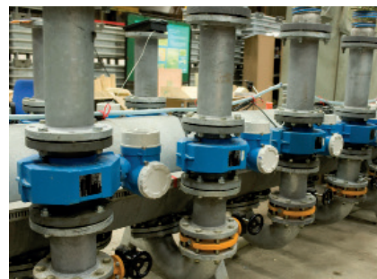
Flow meters and butterfly valves
